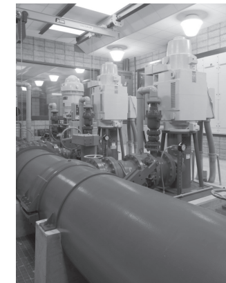
Pictured above is the High Service Pump Room at the Water Filtration Plant. These pumps deliver drinking water to your community
